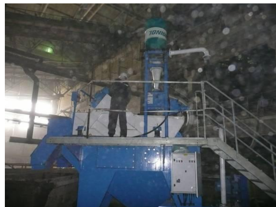
Fig. 5 Fine separation cyclones
