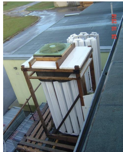
Fig.2. Ventilator above the heat pump evaporator
